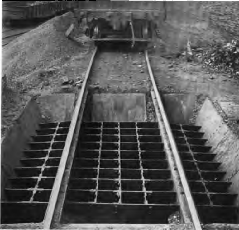
Fig. 1. Grill-Work Protection for Bins, Hoppers, etc.
